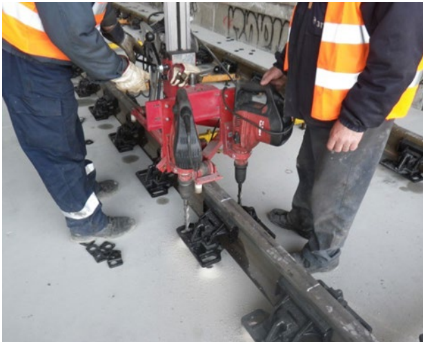
Figure 14: Core drill and glue anchors into the base slab, along with building up the surface with a grout support.
