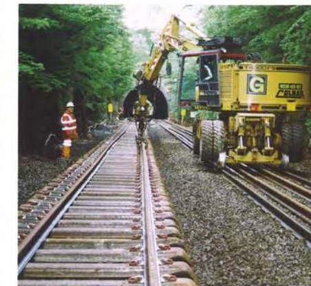
Figure 5 - Rail being installed into FASTCLIP steel sleepers on the Settle to Carlisle line.
