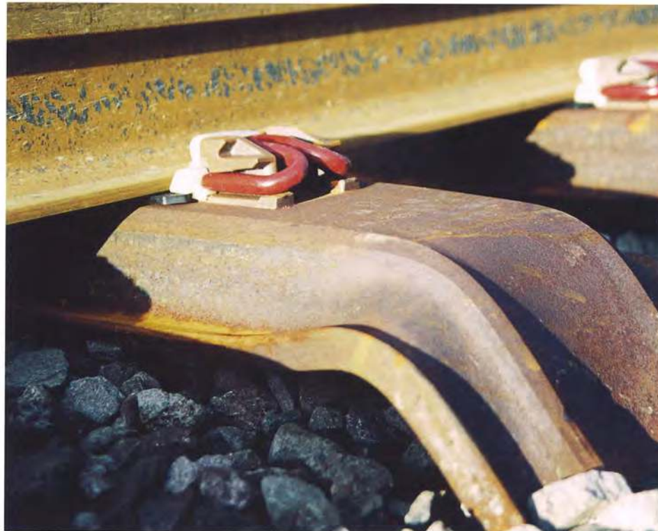
Figure 2 - FASTCLIP attached to steel sleeper by Huck bolt.
