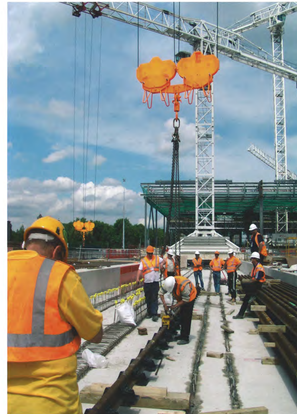
▲ Looking North. Assembled rail with VANGUARD assemblies - about to be craned in to position for final concrete pour (top down construction). Photo by Mark Maher, RLE Senior Track Engineer.
