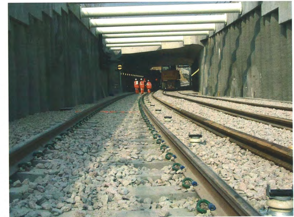
▲ e-PLUS system at Shortlands Junction.
