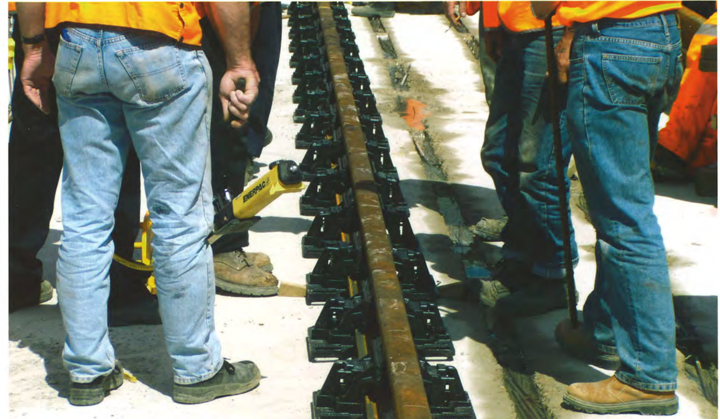
▲ Pre-assembled VANGUARD assemblies on a length of rail waiting to be moved into position, prior to final concrete pour. Photo by Mark Maher, RLE Senior Track Engineer.
