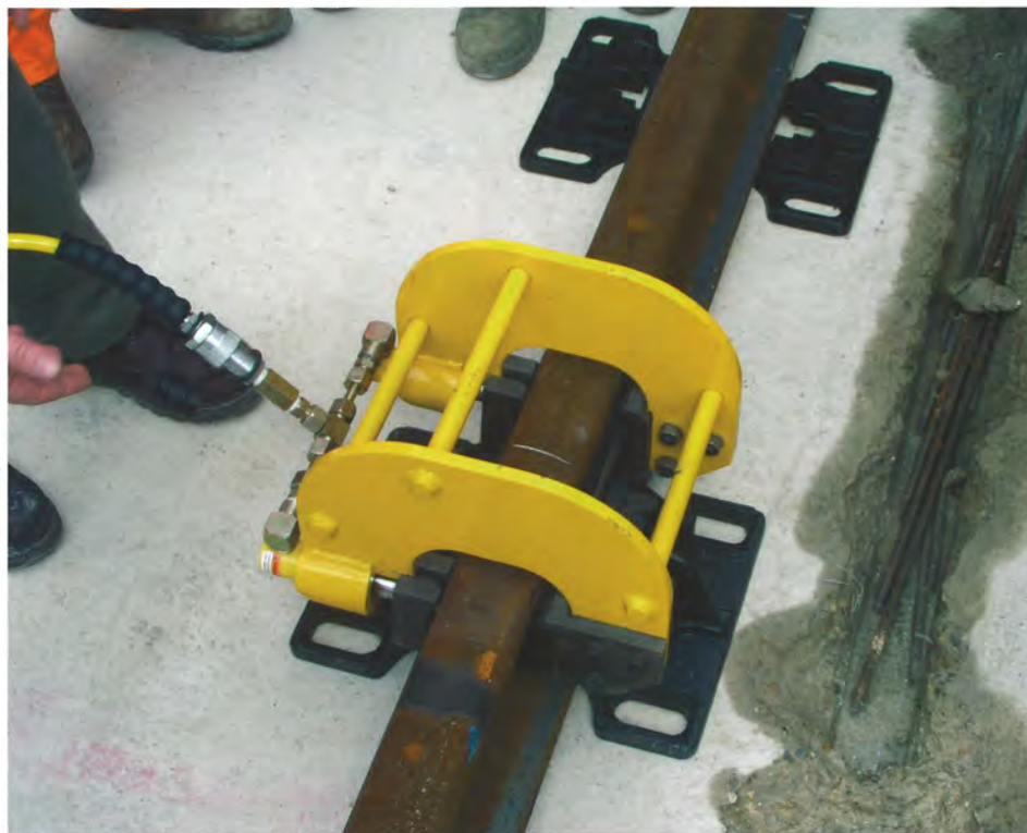
▲ VANGUARD compression tool, used to pre-compress the rubber support elements. Photo by Mark Maher, RLE Senior Track Engineer.
