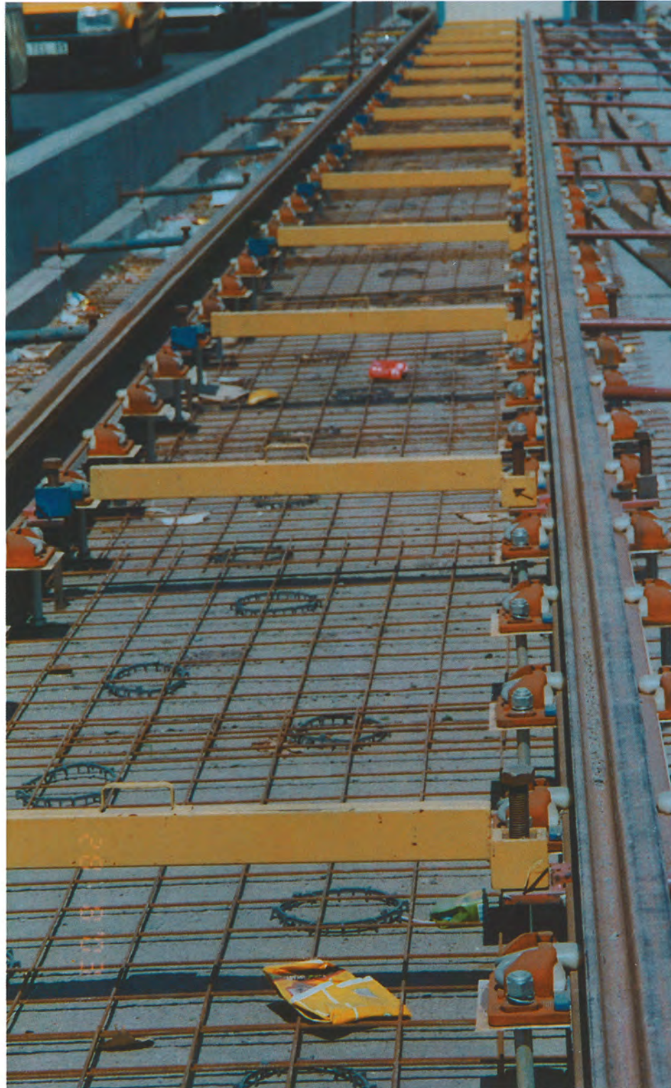
▲ During construction, rails were suspended by support chairs whilst gauge holders provided nominal gauge.
