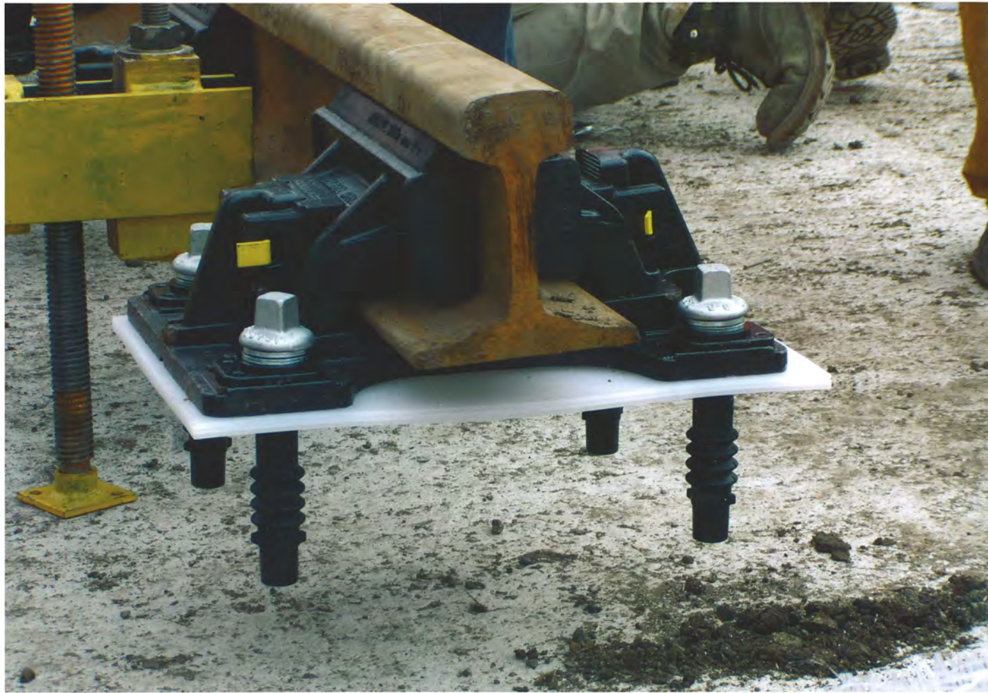
▲ VANGUARD fully assembled on rail, ready to be positioned for top down construction final concrete pour. Photo by Mark Maher, RLE Senior Track Engineer.
