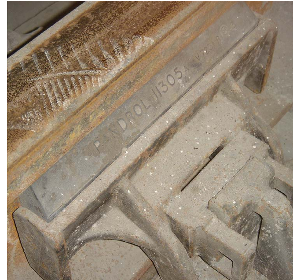
Figure 8 Pandrol VANGUARD installed on Guangzhou Metro Line 3
