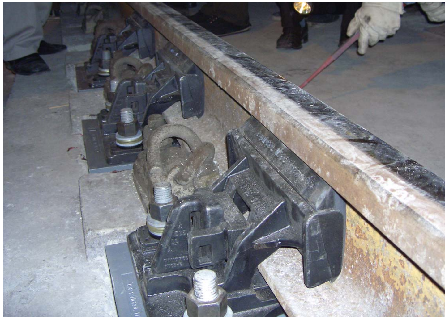
Figure 2 Pandrol VANGUARD installed in a tunnel on Guangzhou Metro Line 1 (Note that conventional fasteners were removed from intermediate positions before measurements were made)
