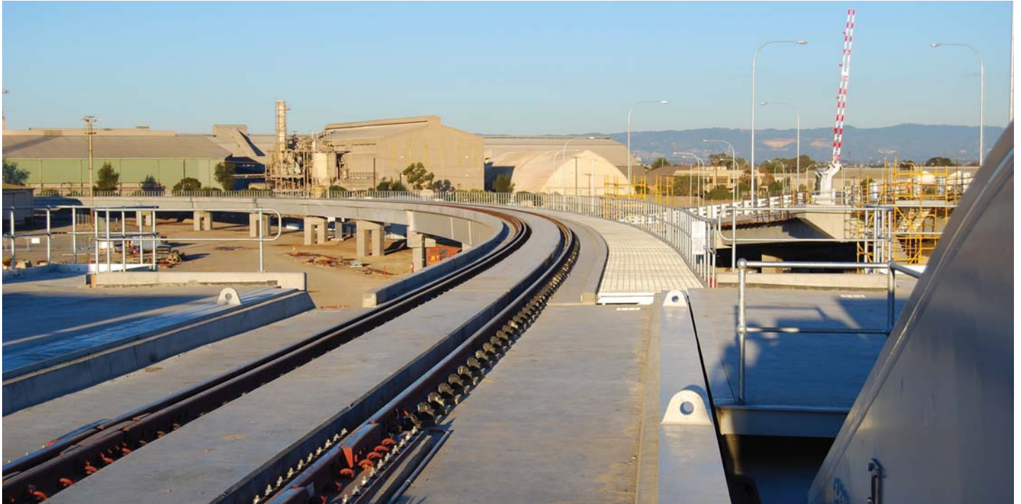
View of the bridge approach to the Bascule section with the mitre joint in the foreground
