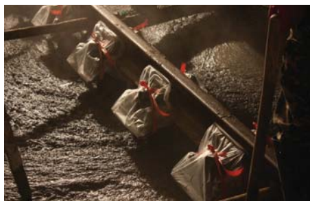
VANGUARD assemblies are protected during the concrete pour to prevent ingress of concrete into the fastening
