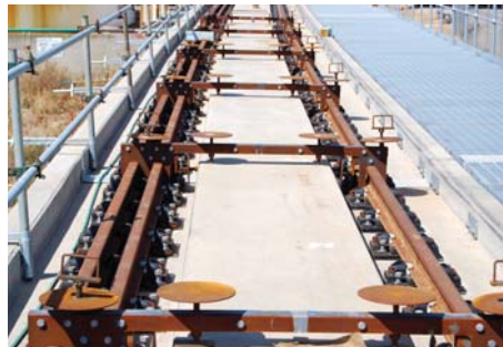
Iron horses used to level and align track Prior to grouting of VIPA-SP assemblies
