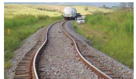
Figure 02 MRS buckled track section and derailed car
