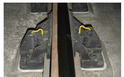
VANGUARD installed on the Beijing Metro
