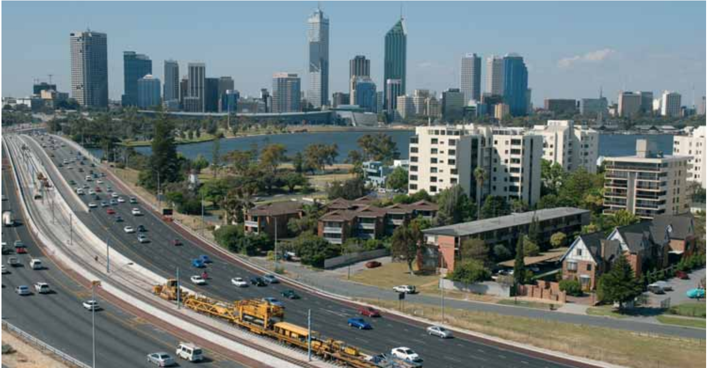
Tracklaying in the median of the Kwinana Freeway (Photo courtesy of PTA)
