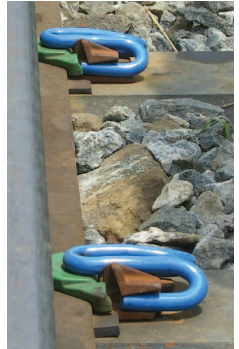
Close up of FD 1408 assembly
