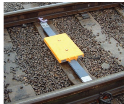
Typical BMS installation for ERTMS
