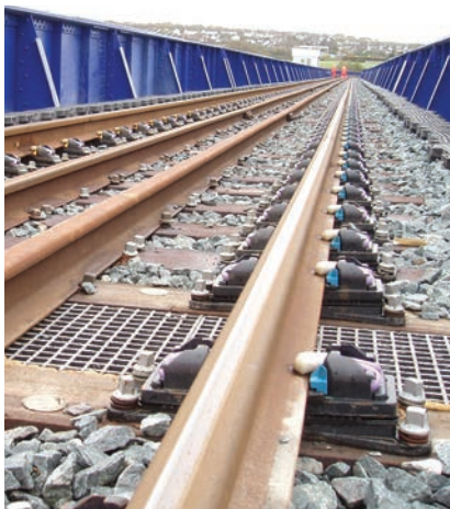
Fixed spans with Pandrol VIPA-SP on timber sleepers in ballast
