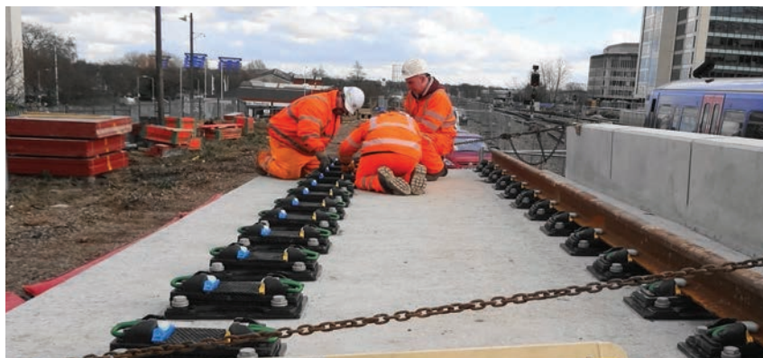
The prefabricated concrete 'lid' during the delivery and training of the installation team
