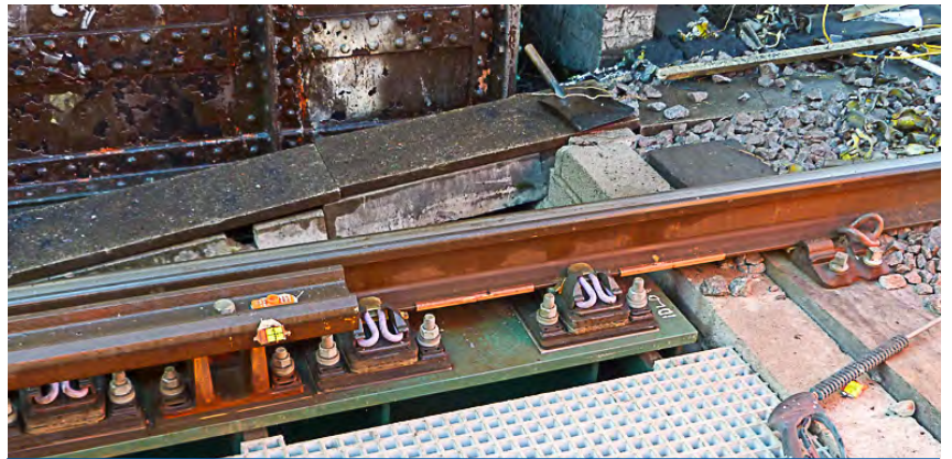
End of the steel beams with VIPA-SP at the abutments into the transition
