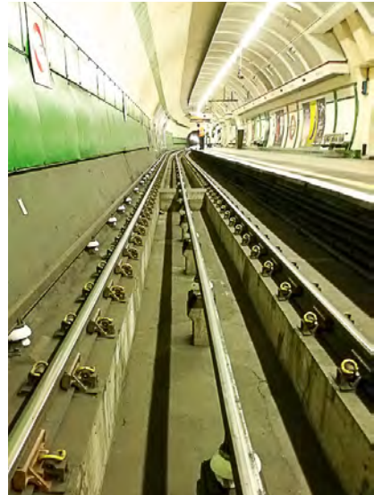
Pilot installation at Maida Vale
