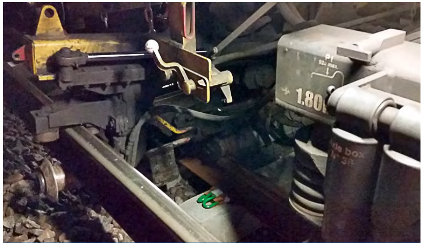
Clipping module behind the old rail, threaded away from the new sleepers with the new rail
