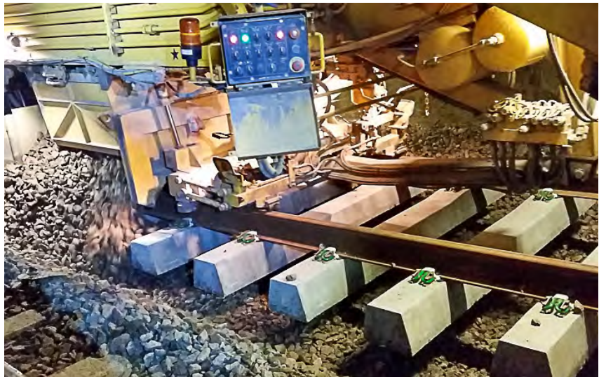
The ballast regulator removes, cleans, replaces and compacts the ballast around the sleepers
