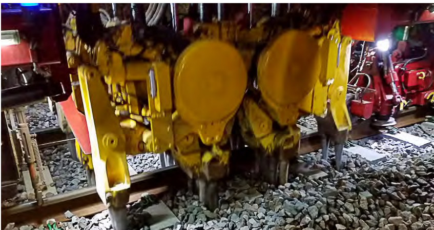
The tamper plunges vibrating tines into the ballast and squeezes the stone under the sleepers
