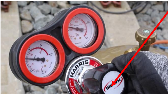
Propane gas line
