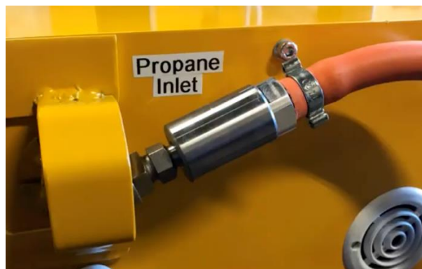
Propane hose connected
