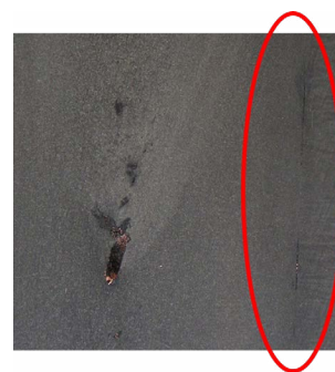
Lack of fusion
